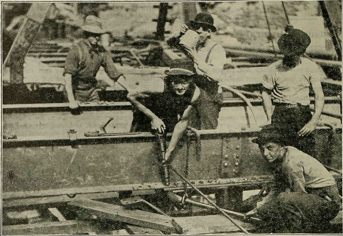
FIG. 1.—PNEUMATIC RIVETER AT WORK ON SUBWAY, NEW YORK. (Cut loaned by Chicago Pneumatic Tool Co.)
