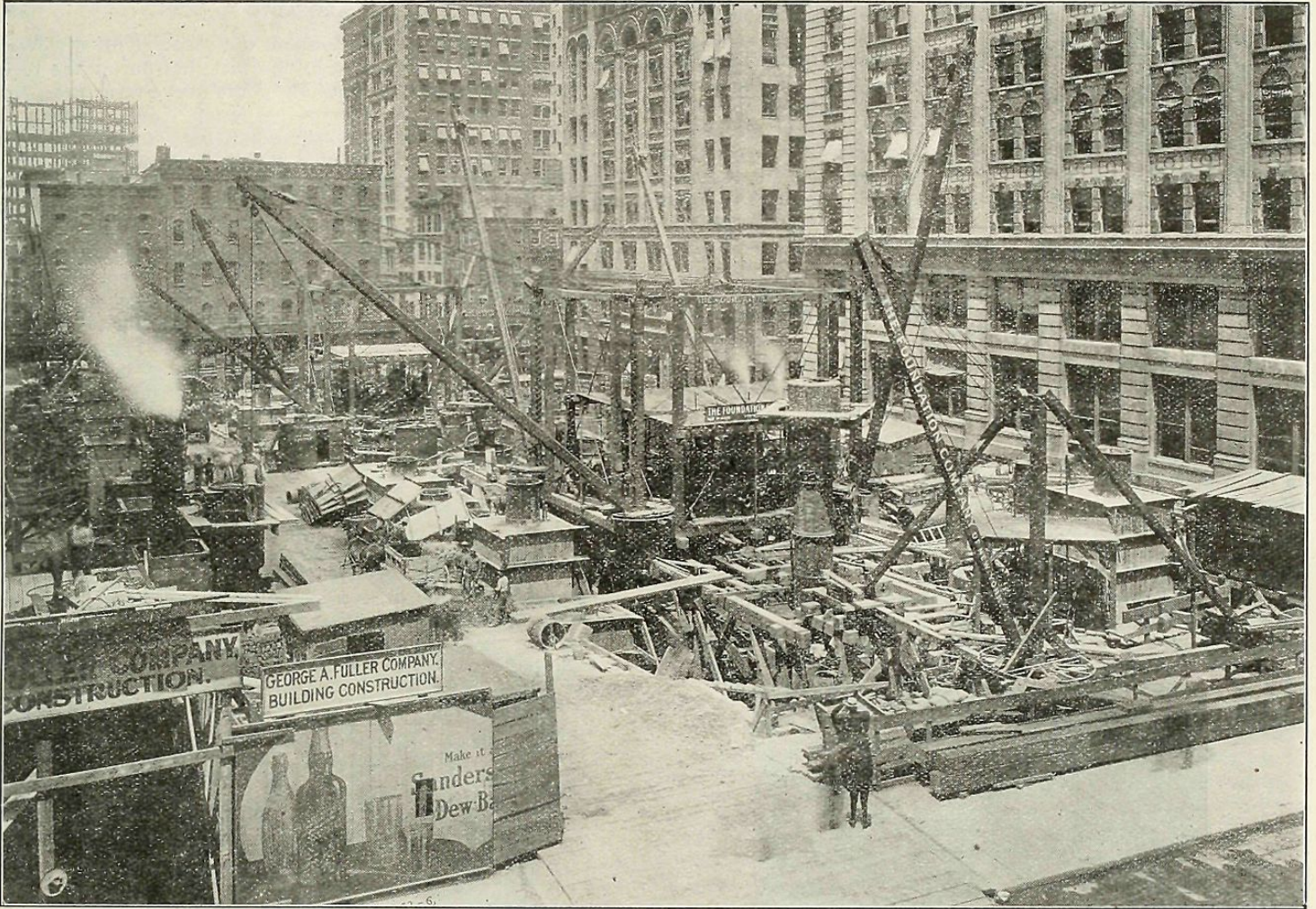
SINKING PNEUMATIC CAISSON FOUNDATIONS FOR THE NEW TRINITY ANNEX AND UNITED STATES REALTY BUILDINGS, 111-115 BROADWAY.
