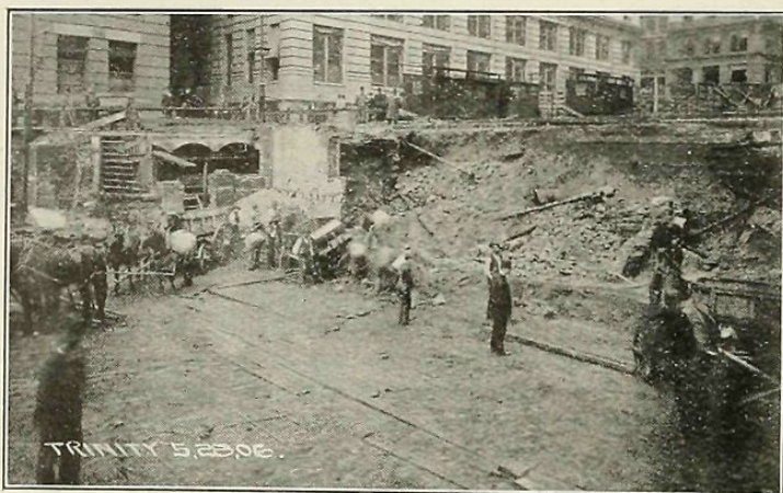
Fig. 1. Making Ready for Laying Foundations of the U. S. Realty Building. May, 1906.
