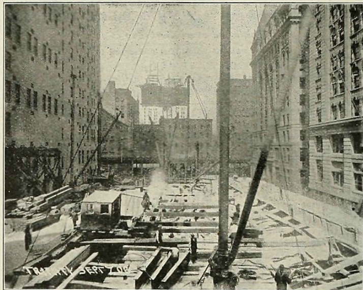
Fig. 2. Foundations of U. S. Realty and Trinity Addition Complete. Preparing for the Structural Steel. September 7, 1906.
