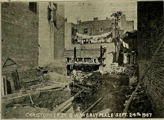
WAREHOUSE AT CHRISTOPHER STREET AND WAVERLY PLACE, NEW YORK, WHICH WILL BE A WINTER JOB.
