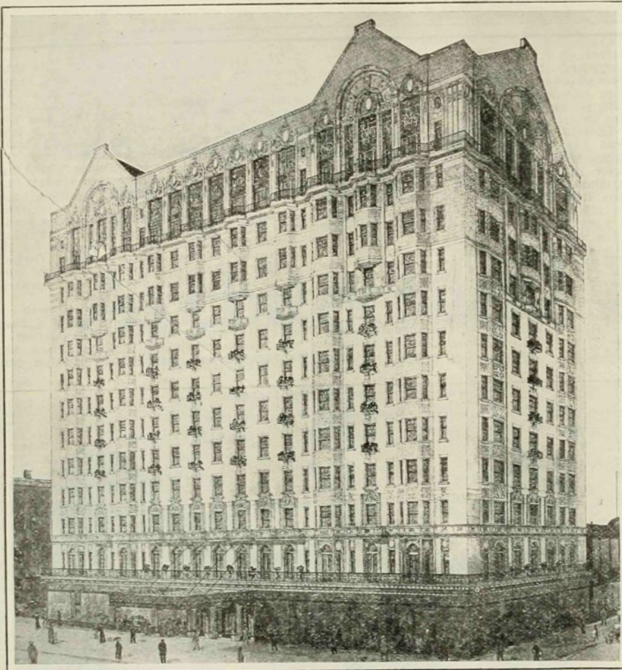
HOTEL THERESE, UNDER CONSTRUCTION AT SEVENTH AVENUE AND 125TH STREET, ON THE SITE OF THE WINTHROP, ONE OF THE CITY'S EARLY APARTMENT HOTELS.
